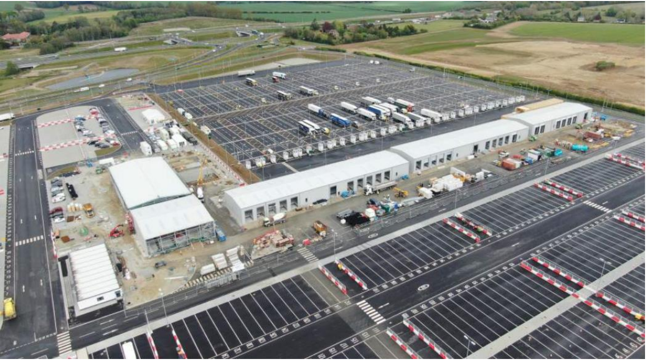
DEFRA sheds under construction. Plant & Produce buildings on the right, two large buildings on left are Animal sheds.
